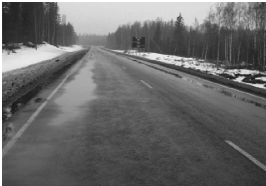
Figure 5. Pooling due to uneven frost heave of fly ash structure in spring 1999.
