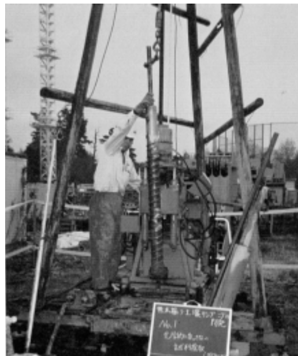
Figure 3. Drilling ability test using the screw-type sampler (Example of a rotary-type boring machine).
