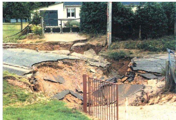
Surface collapse due to underground mining. Lorraine, France
