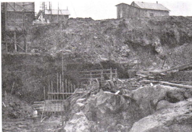
Fig. 1. The excavation for electric plant. The background is section through till and weathered rock and the less weathered granite is seen in the foreground. Photo by K. Virkkala.
