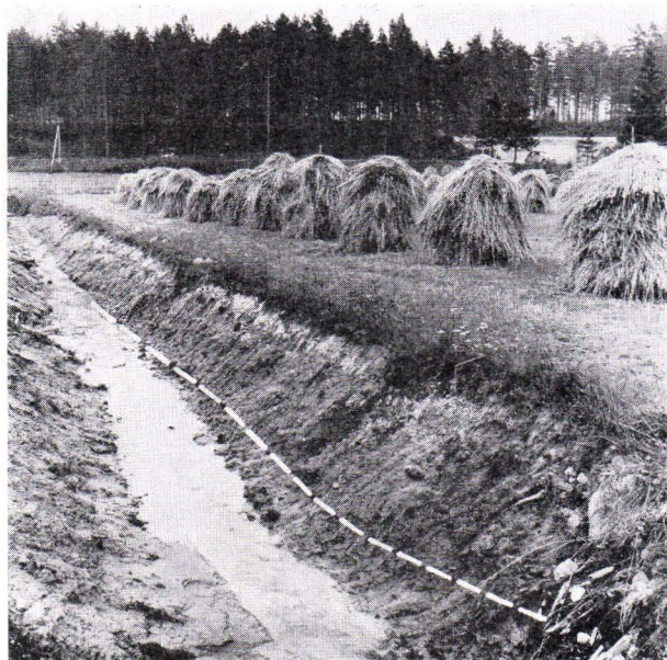
FIG. 6. Ditch dug down to esker layers through clay. Ground water is discharged into ditch. In right background, gravel pit in esker. Siltakylä, Pyhtää.
